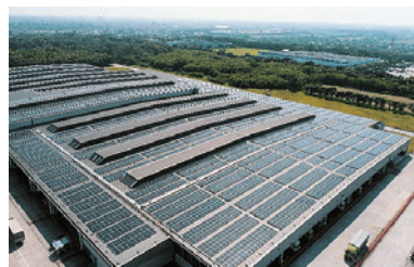
Solar panels installed at TMMIN
